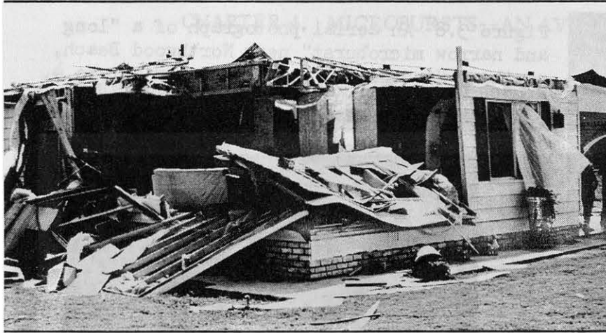
Figure 3.7 An unroofed house in Rosita, Texas. Courtesy of Mr. Antonio A. Dreumont, WSO Brownsville, Texas.
